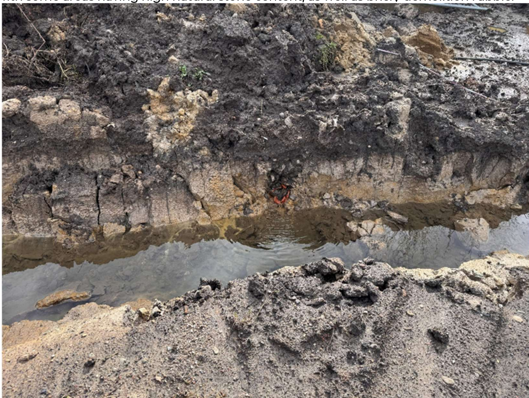
Photo 2: Drainage work (associated with neighbouring housing) on the SE corner of site shows the impervious underlying grey-brown clay that is holding surface water.
