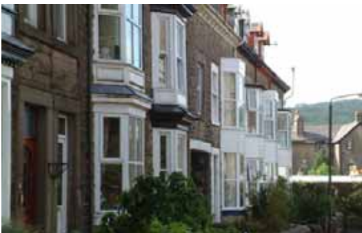
▲ Loss of original joinery to uPVC along Rock Terrace
