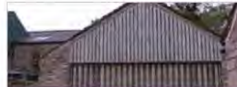
Prefabricated metal buildings do not weather well and remain obtrusive within the landscape. For this reason, materials that do weather well and are sympathetic to the landscape will be preferred. Examples include vertical slatted boarding and painted concrete to blend with existing buildings, reclaimed stone
