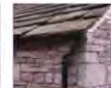
Downpipes and guttering should be discreet, black and located close to the eaves of the building
