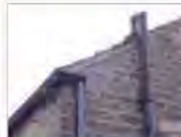
Downpipes and guttering should be discreet, black and located close to the eaves of the house
