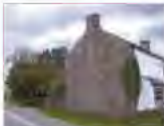
Roofs should be flush to the walls with plain verges and no fascia or barge boarding
